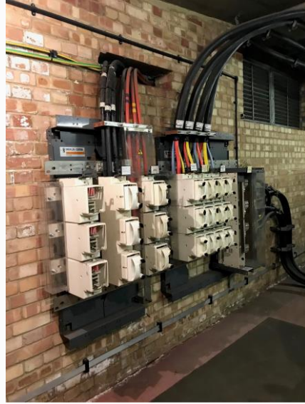
Electrical services LV
